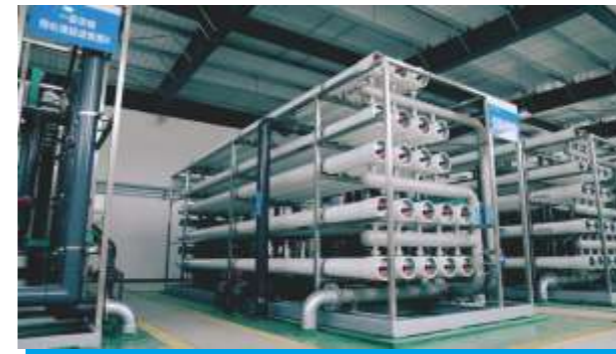
矿井废水零排放 处理量5000TPD
